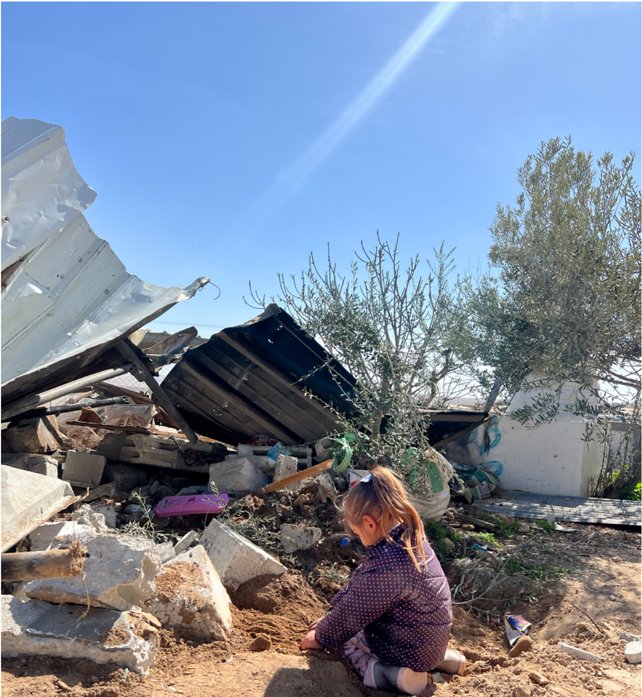
A child kneels in front of a demolished home in Umm al-Khair. Photo: J. Tamimi/WBPC.
