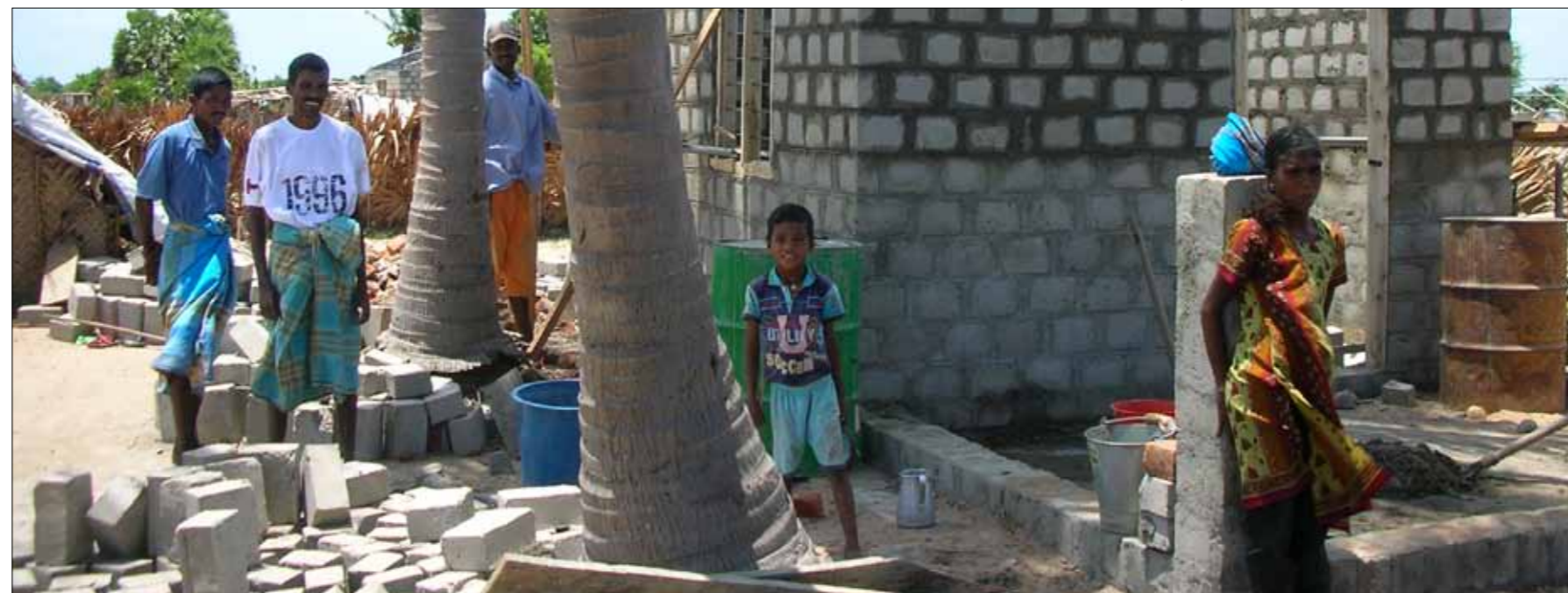
NRC promotes local self-built solutions to shelter needs - ensuring ownership, local design and stimulating local markets. Photo: NRC
