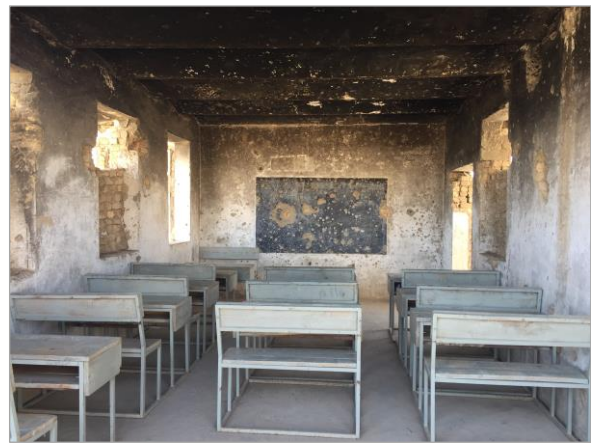
NRC/Andrea Castorina (2018). Photo of conflict-damaged school in Zhari District, Kandahar.
