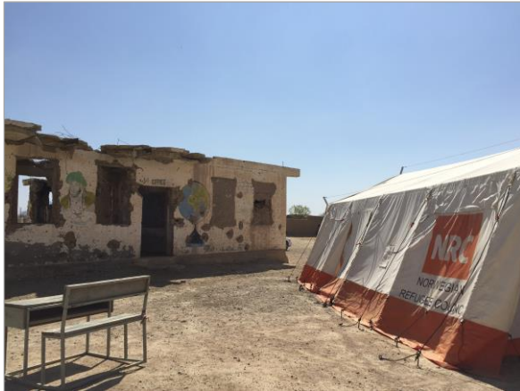
NRC/Andrea Castorina – Conflict-damaged school previously occupied by pro-government militia, now used as an Education in Emergency site for NRC, in Zhari District, Kandahar.
