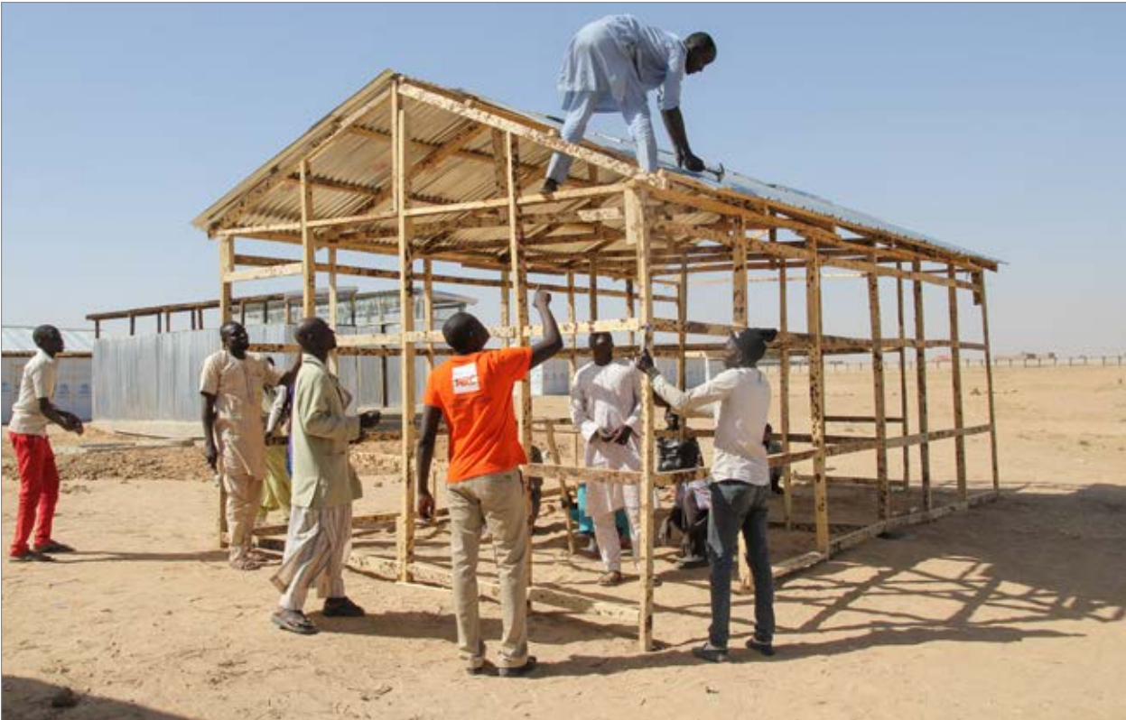
An NRC shelter expert supervises carpenters constructing temporary shelters in Bakasi camp in Maiduguri, Nigeria. Photo: Ingrid Prestetun/NRC
