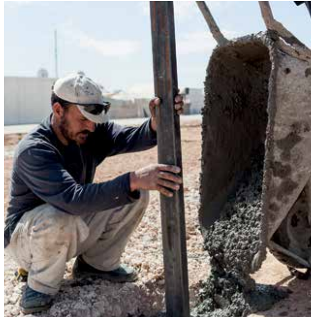
Saddam is a member of NRC's labour scheme. The 34-year-old works with maintenance teams on building a new site at the Zaatari refugee camp in Jordan. Photo: NRC/Christopher Herwig
