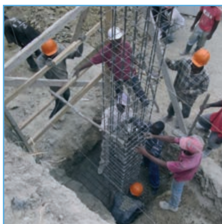
Workers cast concrete on a retaining wall in Morne Hercule. Photo: Jean Julien Dorval/IOM
