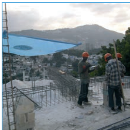
Workers prepare steel reinforcements for a concrete retaining wall in Morne Hercule. Photo: Tanja Bergqvist/NRC
